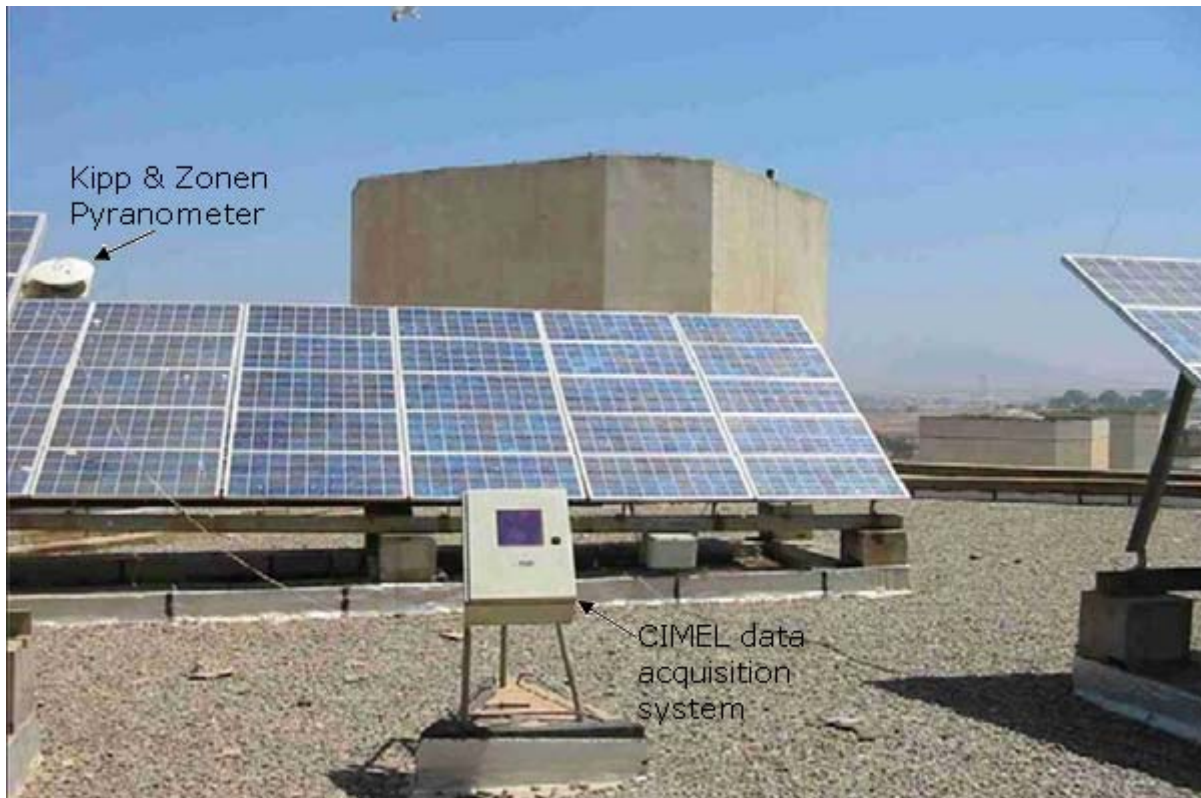
Figure 7.10 PV array insolation measuring equipment on top of roof at University of Science & Technology of Oran.
