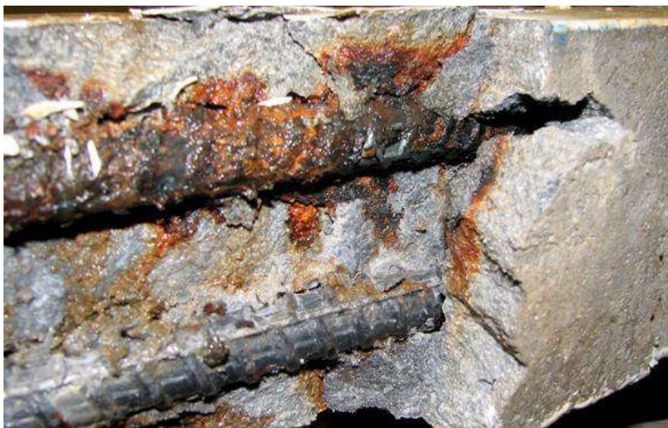
Fig.68. Corrosion des structures
