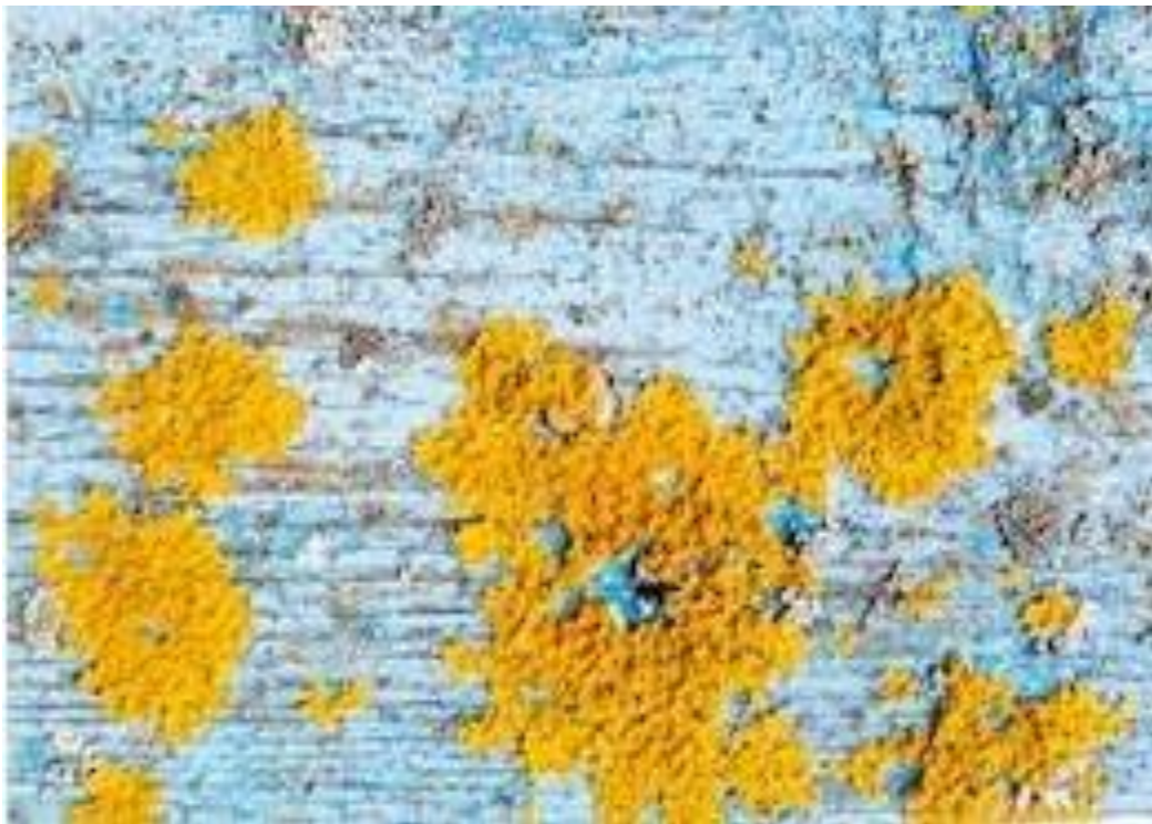
Figure 6 : Photo de la biocorrosion.
