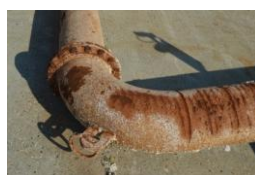
Figure I.29: Corrosion des tuyauteries.
